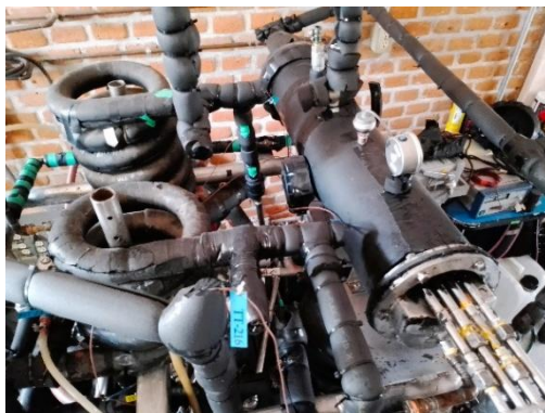
Figure 1. Generator in Heat Transformer
