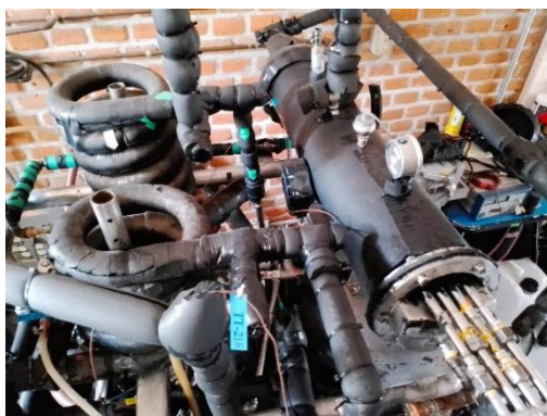
Figure 1. Generator in Heat Transformer
